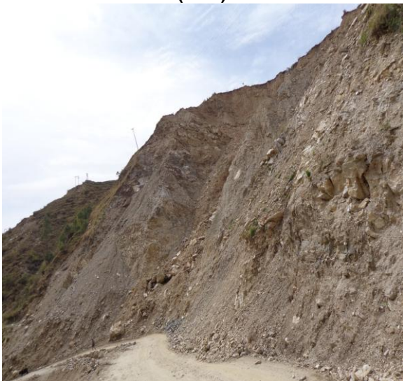
Photograph-4 ; Landslide Near Malla
